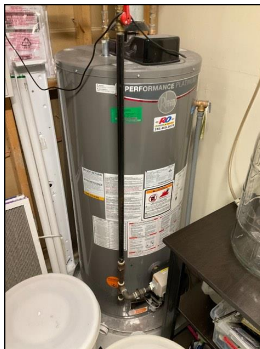
77. Hot Water Tank
