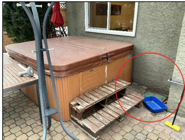
42. Improper slope or drainage
