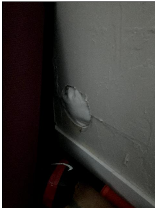
105. Hole in wall
