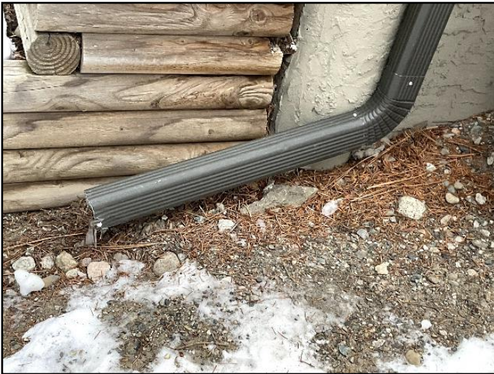
15. Should discharge 6 feet from building
