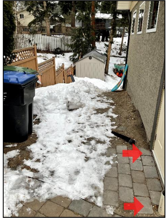
41. Improper slope or drainage
