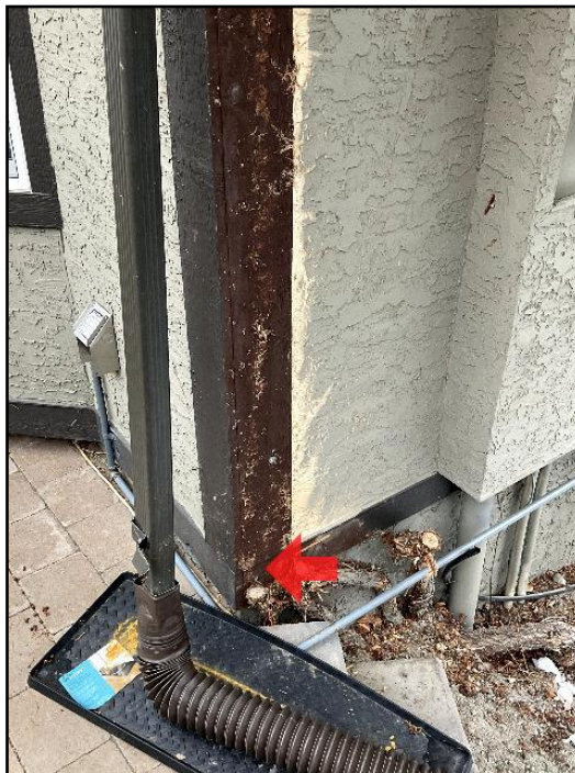
12. Loose gutters down spout
