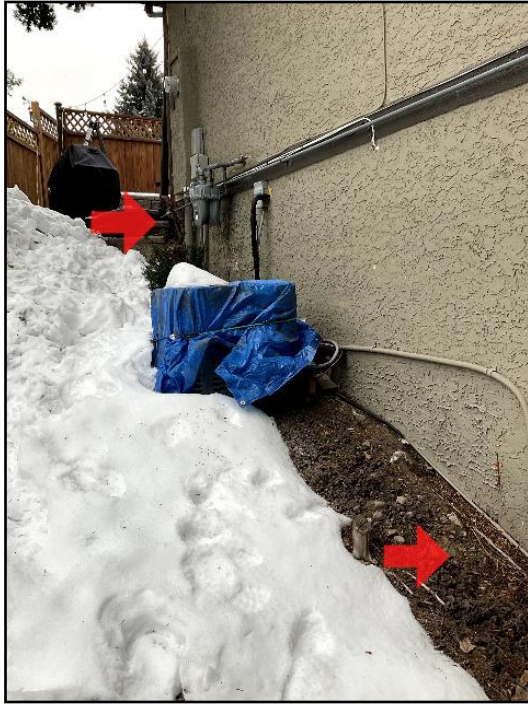
40. Improper slope or drainage
