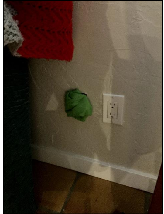
104. Hole in wall
