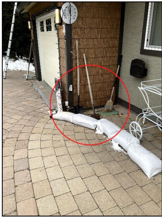
38. Improper slope or drainage
