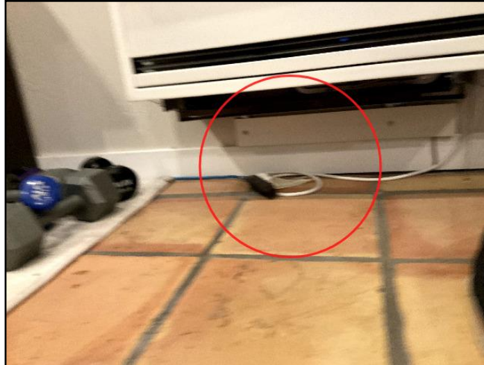
57. Permanent wiring used as extension cord
