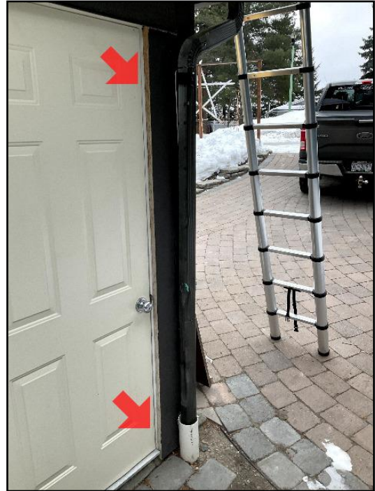
35. Paint or stain needed
