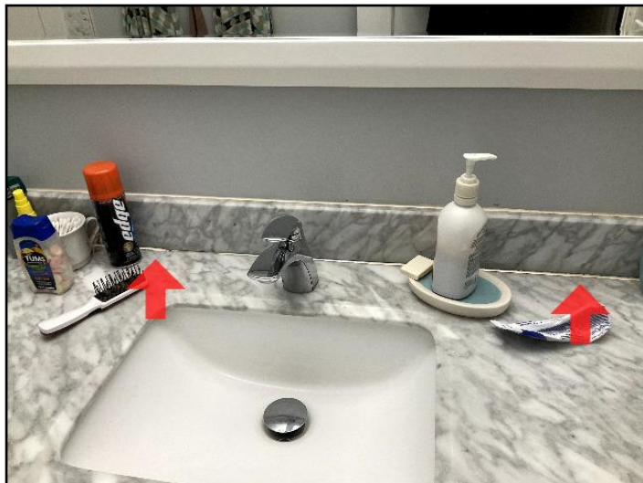
86. Caulking loose, missing or deteriorated
