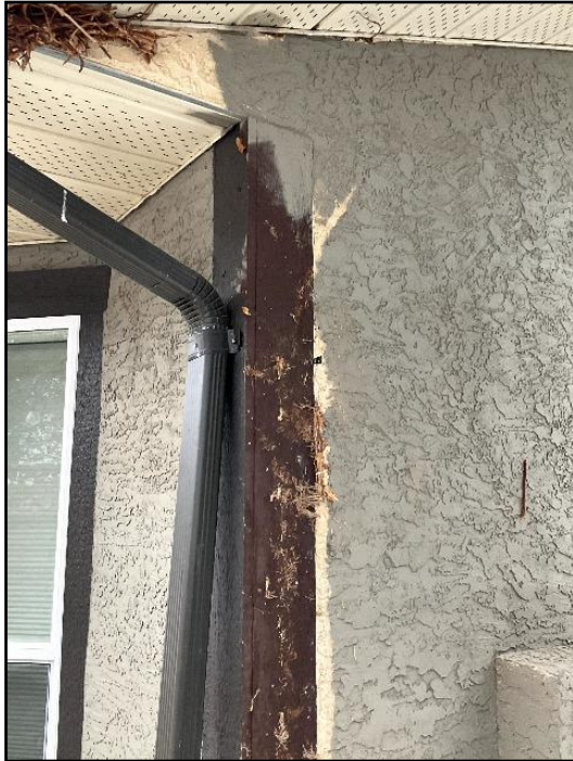
34. MePaint or stain needed mechanical damage
