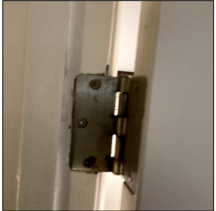
109. Loose or poor fit
