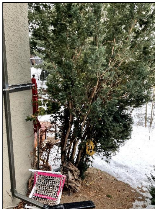
37. Trees or shrubs too close to building
