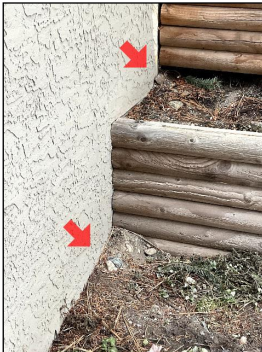
24. Too close to grade
