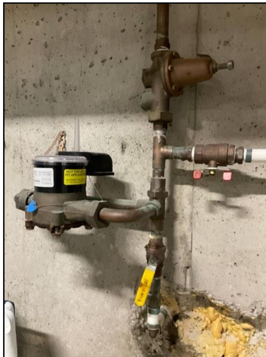
79. Main Water Shut Off
