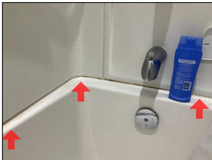
87. Caulking loose, missing or deteriorated
