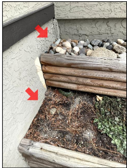
23. Too close to grade
