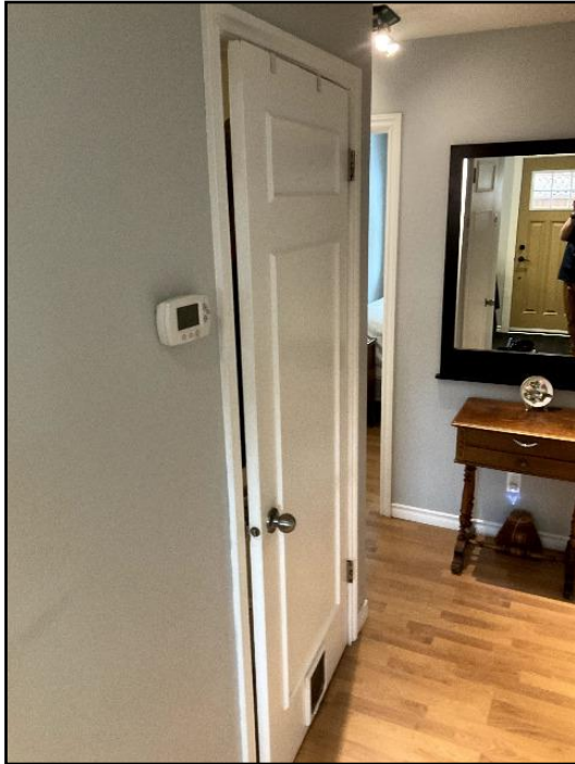
108. Loose or poor fit
