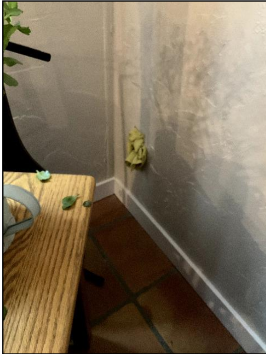
103. Hole in wall
