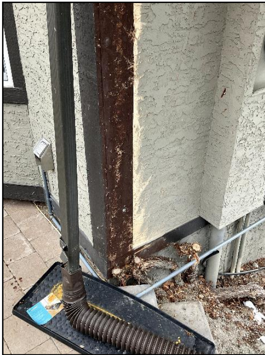
13. Should discharge 6 feet from building
