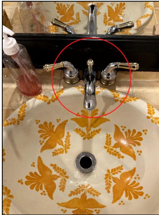
84. Loose taps and faucet
