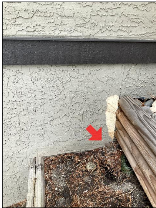
22. Too close to grade
