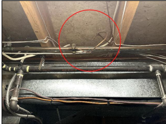
56. Copper - water pipe
