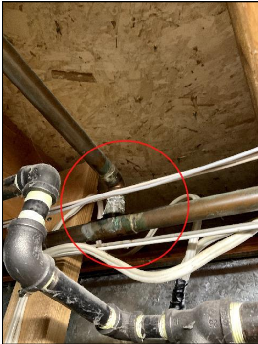
82. Corroded copper pipe
