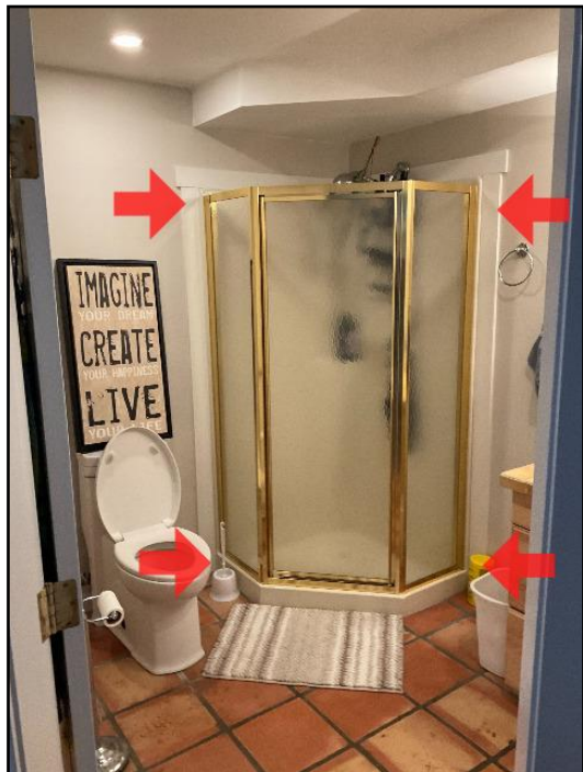
85. Caulking loose, missing or deteriorated
